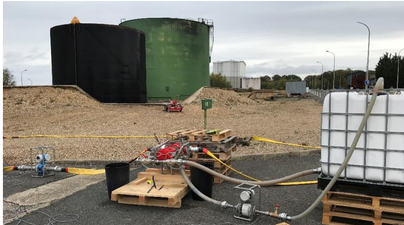
Figure 5.5. Setup of Firedos proportioner with flow meters used during Phase 2 tests
