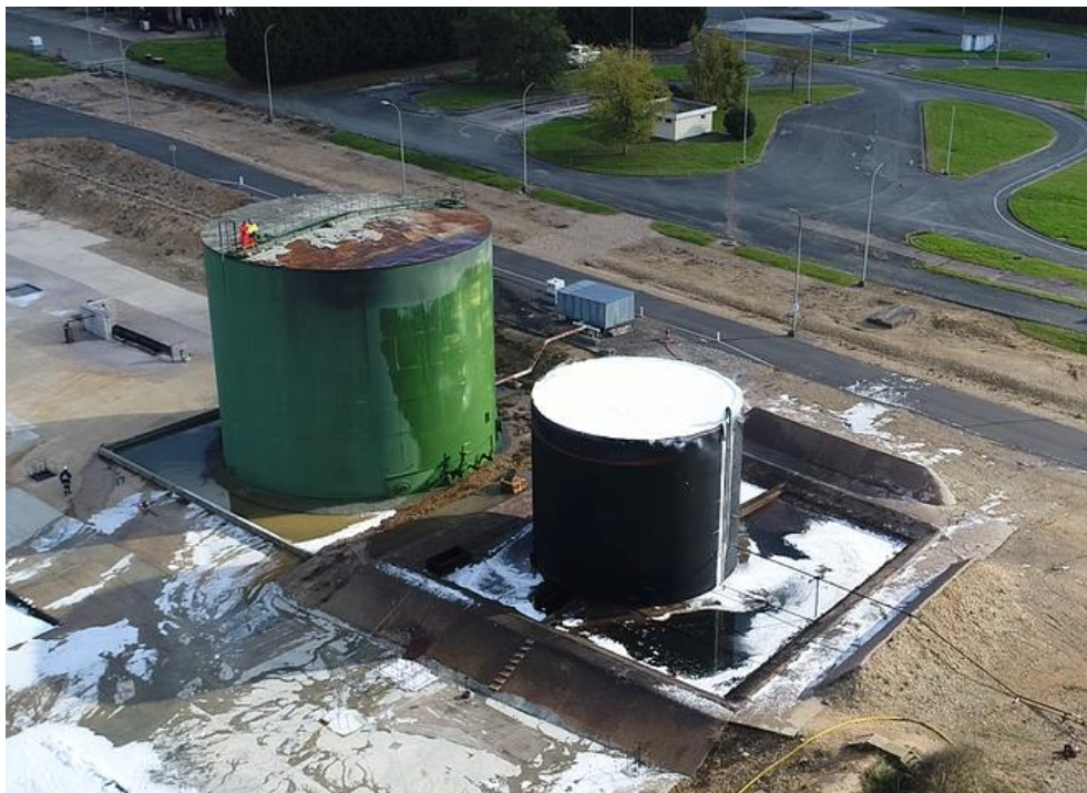
Fig. 10 Fire extinguished. Note steam from edges
